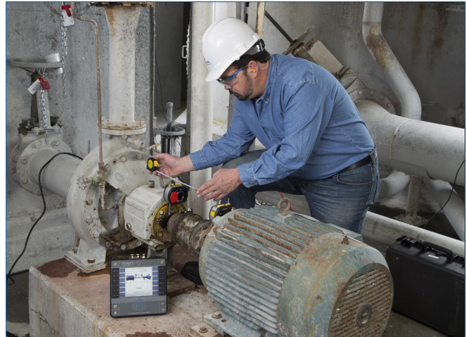
Laser alignment and precision balancing jobs can be stored and reported in AMS Machinery Manager.
